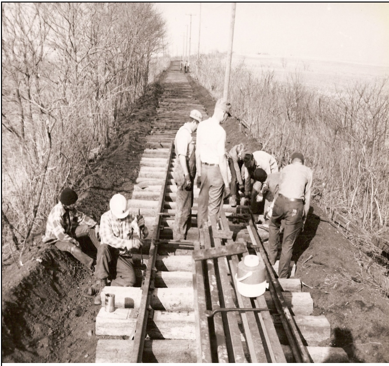
Work is underway to lay track northwards toward White Heath in the winter of 1973. Dave Mann and members are about half way up the “Hill” on the former IT right of way.
