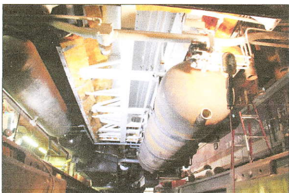
One of two water tanks reinstalled under the diner. Note new steel water tank supports and entire area above/around tanks painted white to protect the steel from further corrosion and to make work inside the water tank enclosure easier to see in the future.
