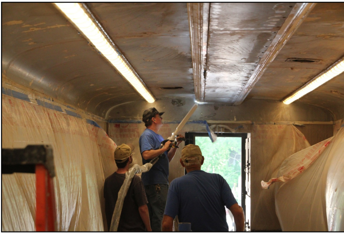
Kirk Reynolds, Dennis Slone, and Paul Bundy work at dry ice blasting aluminum trim, and residue from the chemical stripper.
