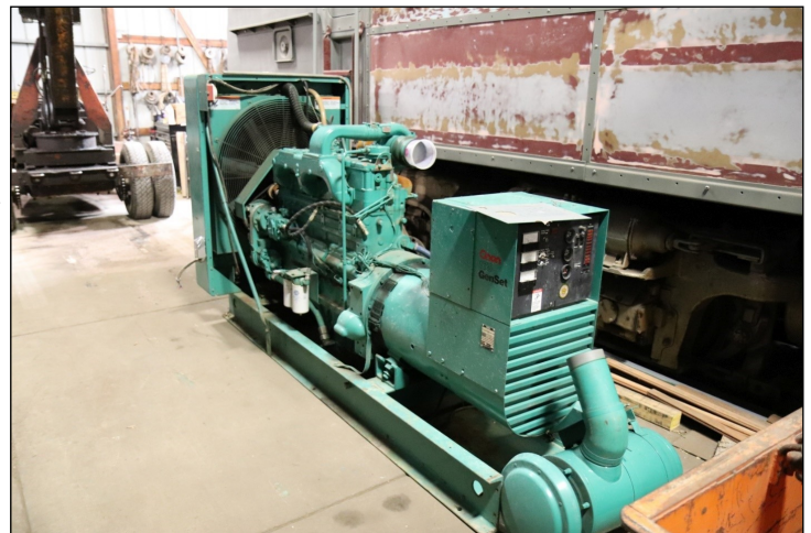
New Onan 175 KW Generator for our head-end-power.
